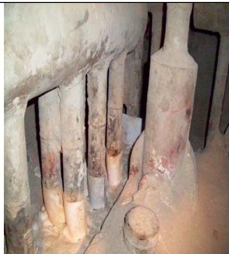
Prepared tube penetration with 2mm thermal insulation paper adhered to the tubes with Maxigrip adhesive (rated 1000degC) for expansion allowance. Bio-soluble blanket layed down to prevent loss of refractory material through the Penthouse floor
