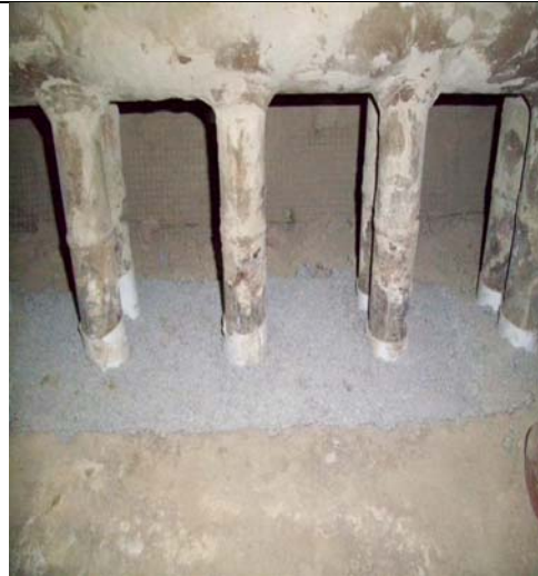
Completed area of Thermbond Formula 3L castable repair showing the thermal insulation paper wrapped around the tubes.
