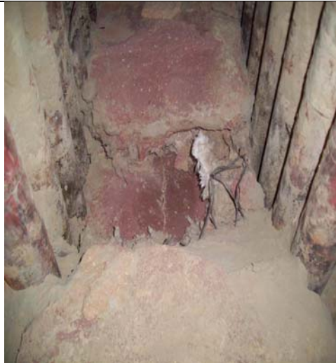
The Boiler penthouse floor was badly eroded. A heavy layer of fly ash dust was removed by vacuum, all loose broken refractory removed before the Thermbond refractory repair commenced.
