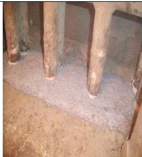
Completed area of Thermbond Formula 3L castable repair, there were 137 tubes repaired on this outage and the remainder would be done on the next outage.
