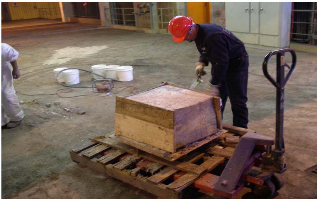
November 2006: Thermbond Formula 6L precast door block for boiler furnace.
