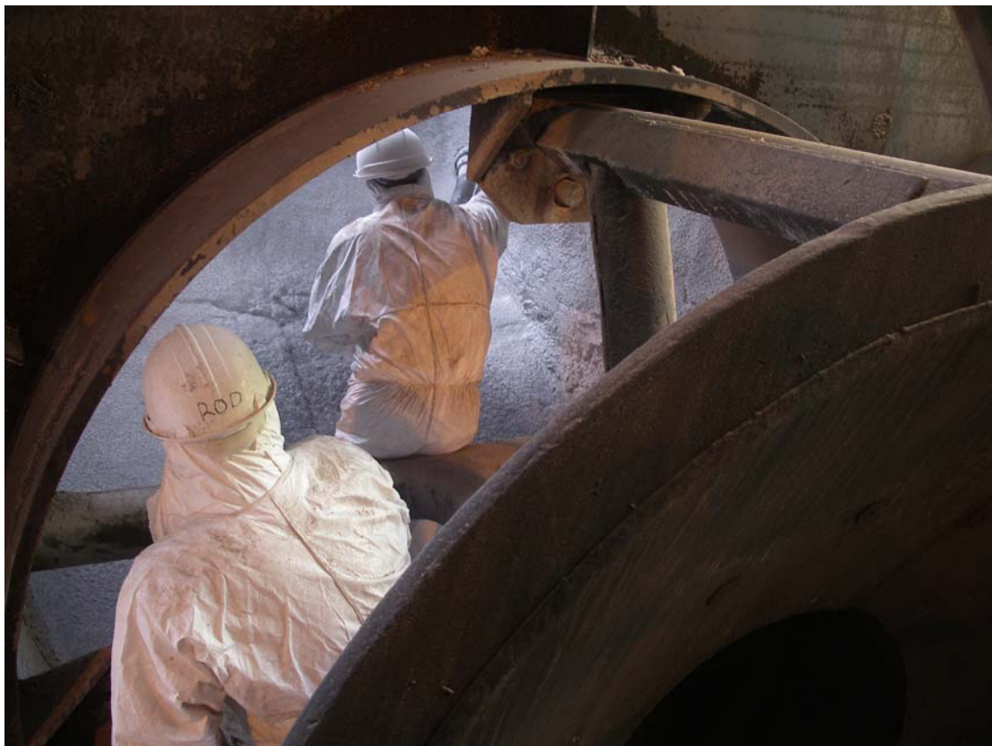
November 2006: Contractor Andreco Hurll spraying Thermbond Formula 6AG gunnite, showing low dust emission and minimal rebound during gunning operation.
