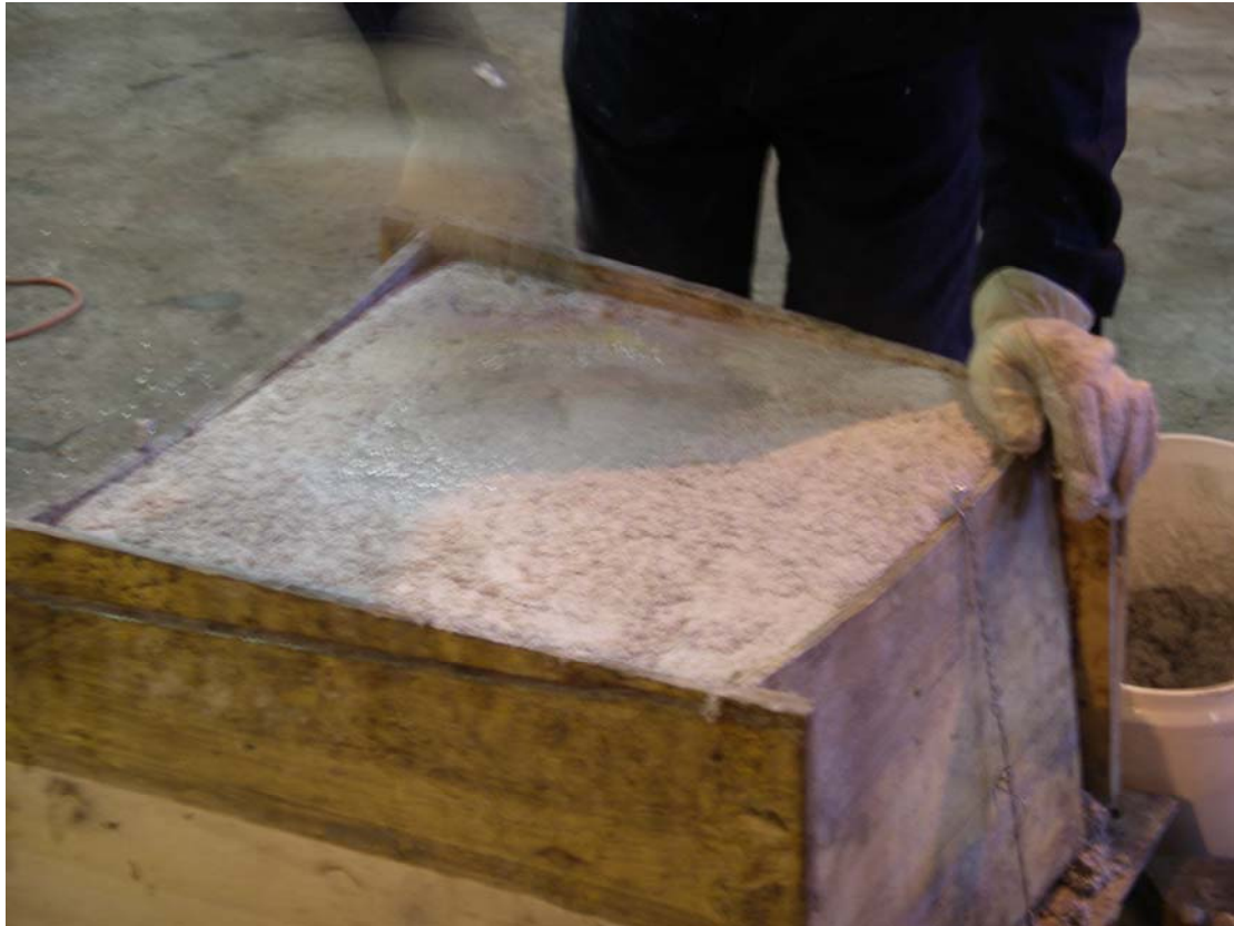
November 2006: Thermbond chemical bond castable precast boiler door block. Andreco cast Thermbond Formula 6L door block into timber mould.
