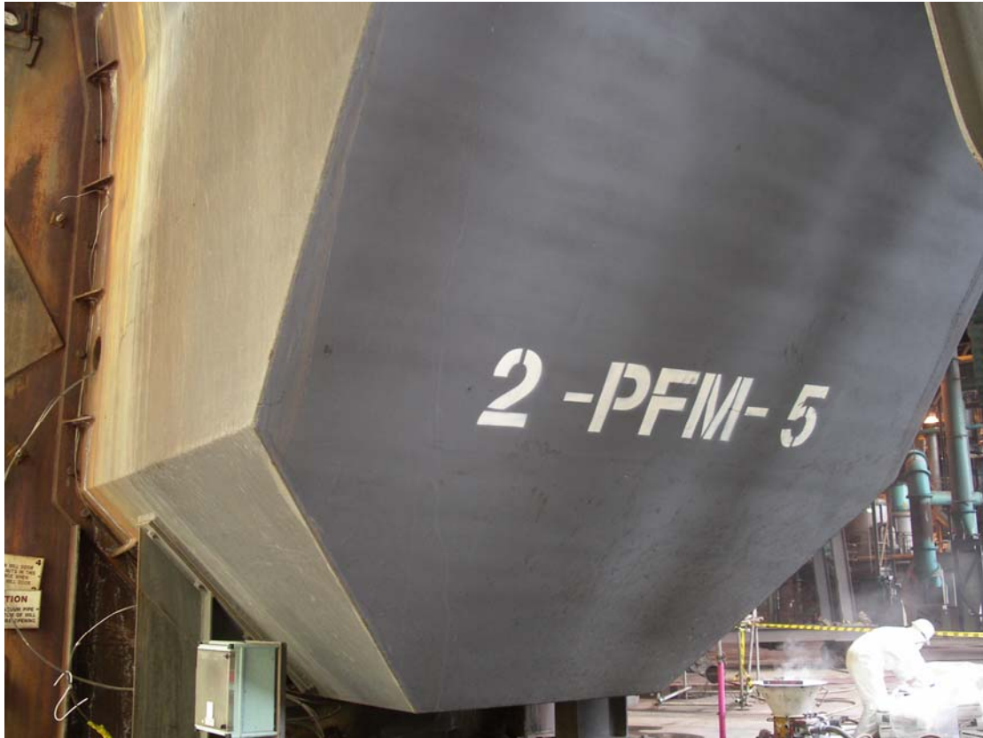
November 2006: Loy Yang Power Mill door Thermbond gunning repairs. Thermbond Formula 6AG gunning castable installed to repair fired refractory.
