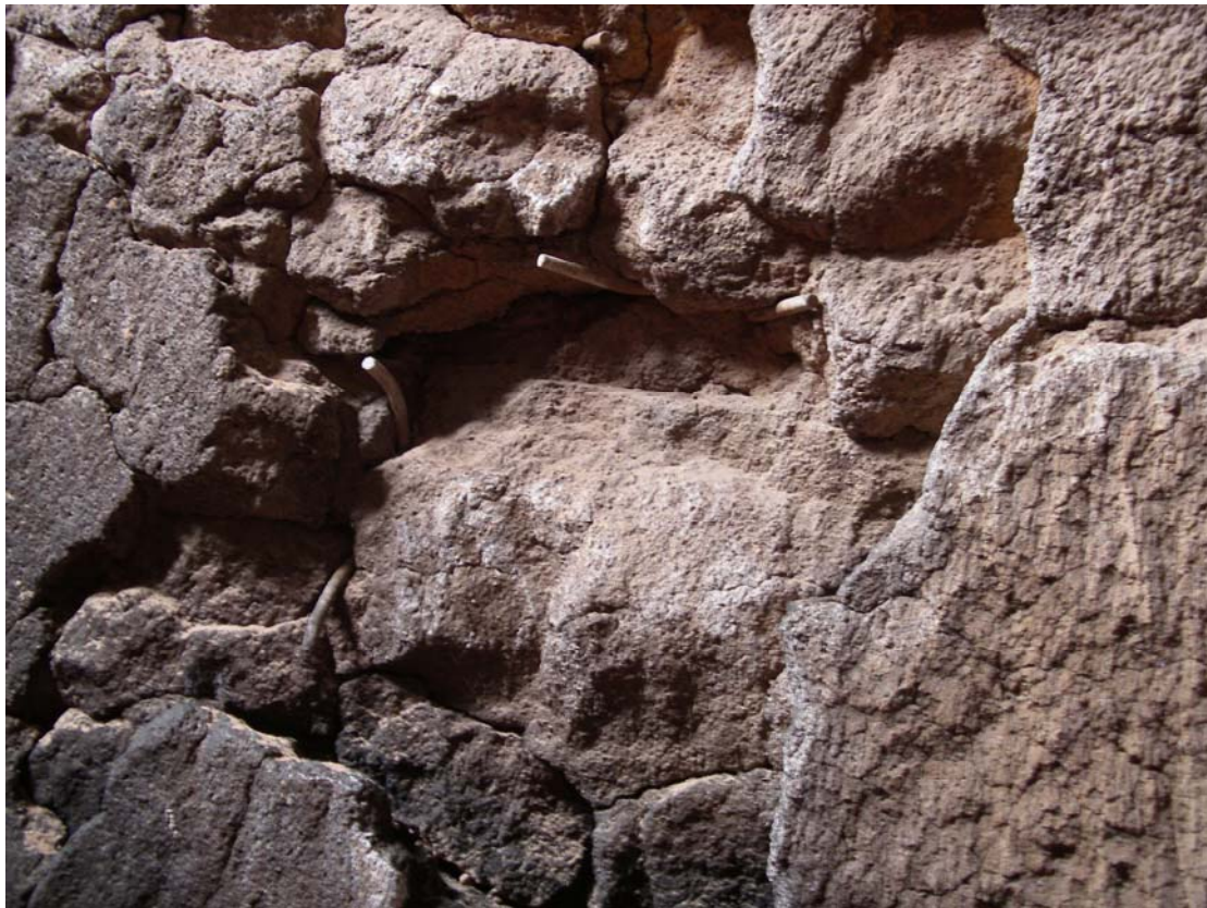
November 2006: Condition of Loy Yang Power mill door fired refractory before Thermbond F6AG castable gunned onto mill door fired refractory.
