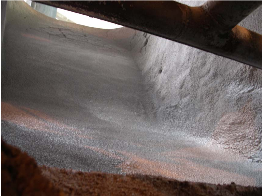
November 2006: Result of spraying 48 bags Thermbond Formula 6AG gunning castable onto fired, cleaned refractory in Loy Yang Power 2-PFM-5 boiler mill door.
